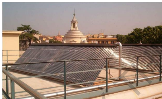
Evacuated tube collectors - ETC [2]
