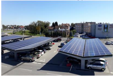
Photovoltaics in parking lots[1]
