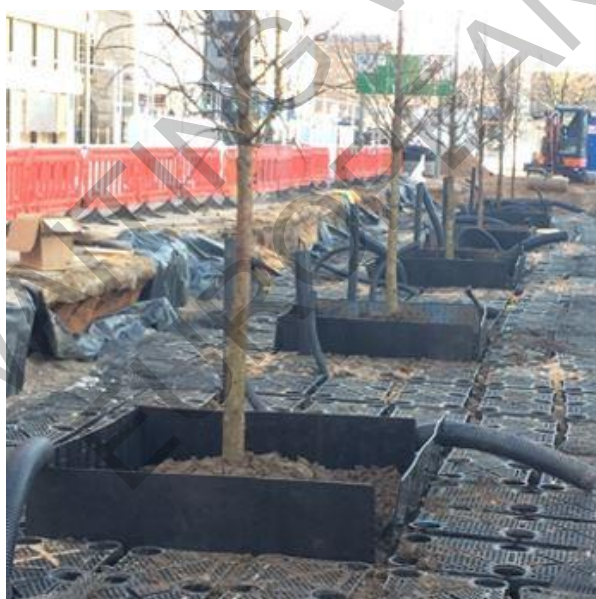
Urban Catchment Forestry (SuDS). Source: URBAN GreenUP (H2020 Project GA No 730426) and Liverpool City Council
