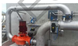
PaT (Pump as a turbine)
