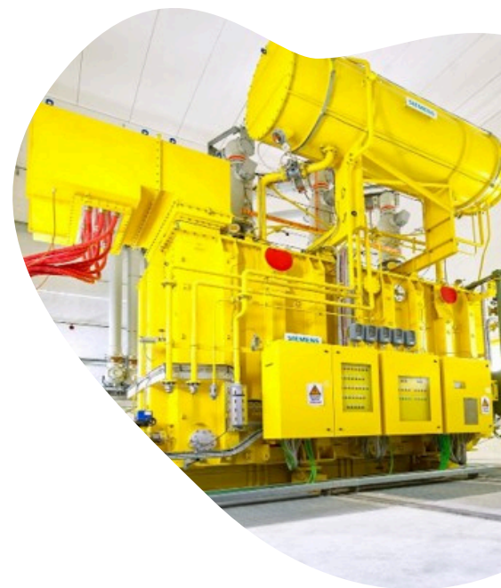
Arbarello HV-MV Primary Substation
